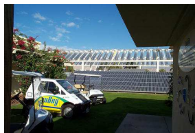
Solar-powered electrolysis system at SunLine Transit Agency
